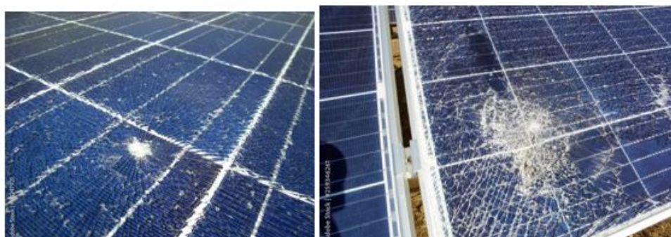
Fig. 2 Sample overhead images of Solar Panels with cracks
